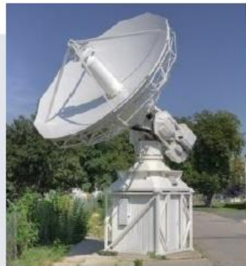
Groundstations for Satellite Communication
